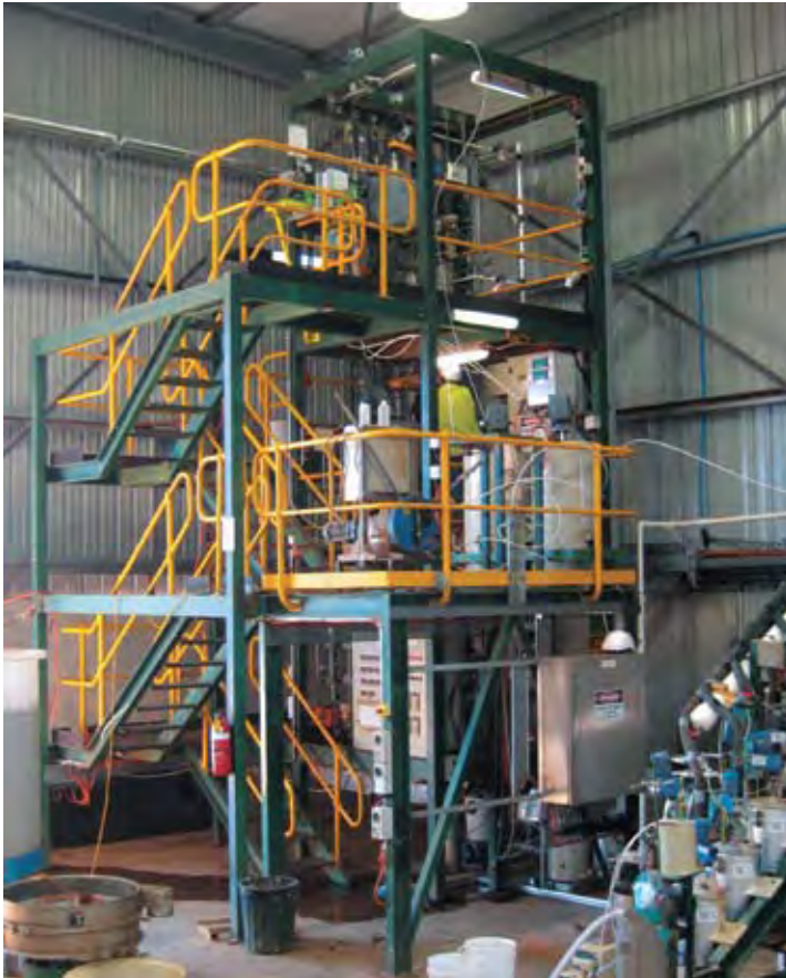
Figure 2: Continuous 4 Pot Pilot Plant.
